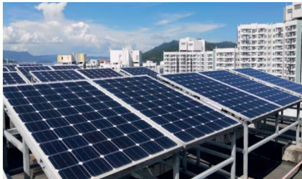
The solar energy generation system installed by the Housing Authority at public rental housing estates
